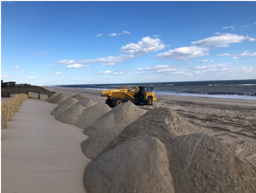
Seaview purchased sand from the County to build the beach and dunes higher on the east end of the community, which was not part of west end repair project (Photo Luke Kaufman)
