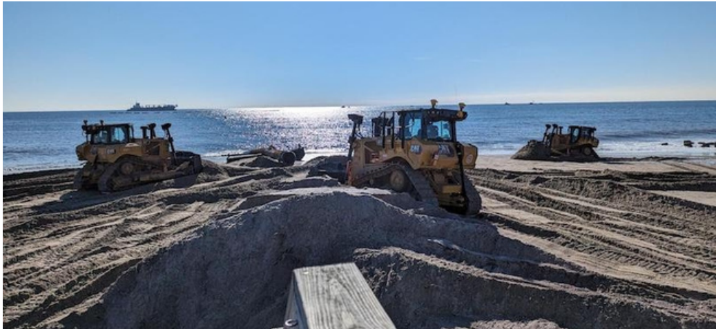
GLDD earth moving equipment shaping the dredged sand into new dunes and a wide berm for the Village of Ocean Beach (Photo Theresa Macri)
